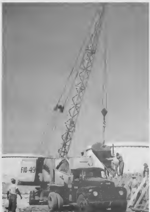
FOUNDATIONS ARE poured into the wooden forms. The concrete ring, when completed, stood eight feet high FUNDESHINAN ta wòrdè hasá den e formanan di pila. E renchi di concreto, ora e ta cla, tabata ocho pia halto.
